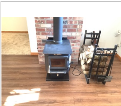
Reference picture of the freestanding wood stove in the basement
