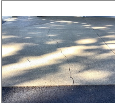
The driveway appeared to be in overall usable condition. Typical cracks were observed at the concrete driveway. Recommend sealing cracks to prevent further deterioration.
