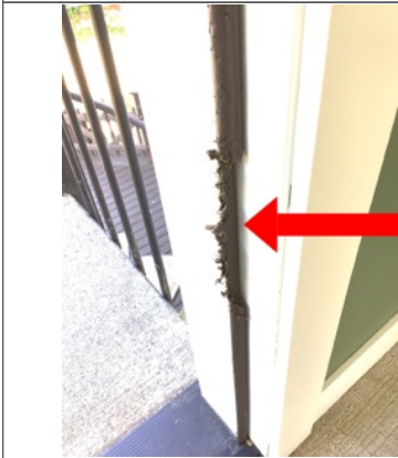
Summary item 1i Damaged/torn weatherstripping was observed at the upper west facing exterior door at the top of the spiral staircase. Recommend repair or replacement of the damaged/torn weatherstripping as needed.
