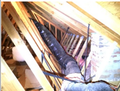
Roof/attic framing, roof sheathing and insulation appeared to be in overall functional condition where accessible.
