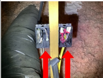
Summary item 7 Open electrical junction boxes were observed in the attic north of the attic access. Recommend installation of cover plates at any/all open electrical junction boxes.
