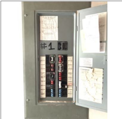
Reference picture of the electrical panel box.
