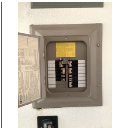
Reference picture of the electrical sub-panel
