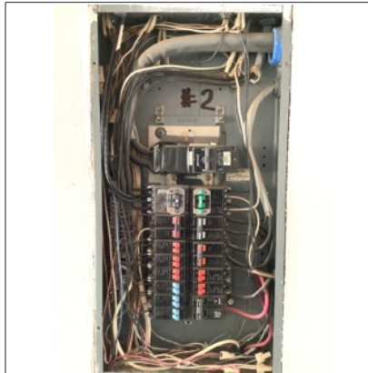
Interior image of the electrical panel box/wiring.
