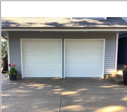
The overhead garage door(s) appeared to be in overall functional condition unless noted
