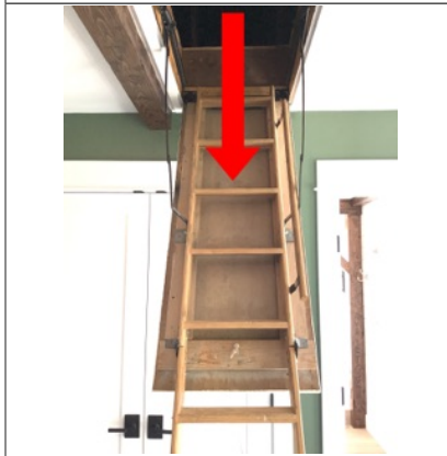
Summary item 1k No insulation was installed at the attic access panel/pull down ladder in the Primary Bedroom. Recommend installing insulation at the top side of the attic access panel to prevent heat loss if deemed necessary.
