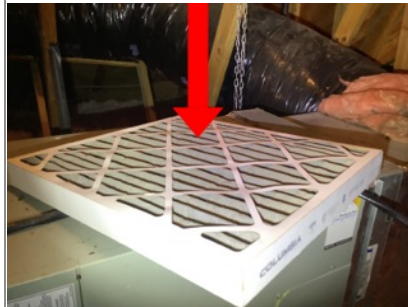
Summary item 6 The air filters in both HVAC systems were dirty at time of inspection and should be replaced. It appeared that the systems had not been serviced since approximately 09/2020. Recommend general service/cleaning of the HVAC equipment by a licensed contractor if deemed necessary.
