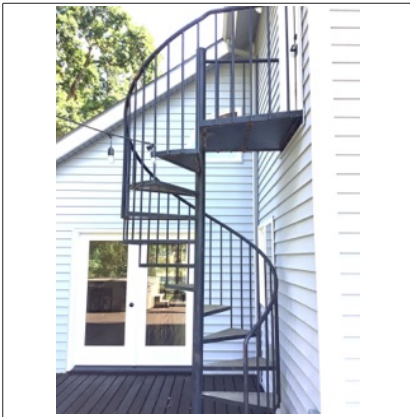
The exterior steps appeared to be in overall usable condition at time of inspection.
