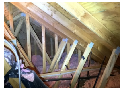
Roof/attic framing, roof sheathing and insulation appeared to be in overall functional condition where accessible.
