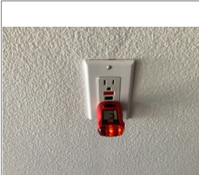
The electrical outlets in the garage are GFCI protected and appeared to be functioning properly at time of inspection
