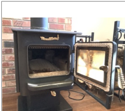
The freestanding wood stove appeared to be in overall usable condition based on a visual inspection only. Flue could not be fully examined so no representation could be made.
