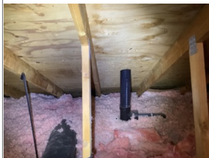
Roof/attic framing, roof sheathing and insulation appeared to be in overall functional condition where accessible.
