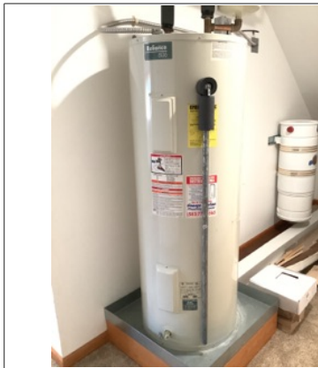
Reference picture of the 80 gallon electric water heater
