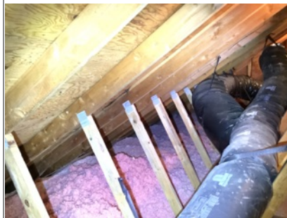
Roof/attic framing, roof sheathing and insulation appeared to be in overall functional condition where accessible.
