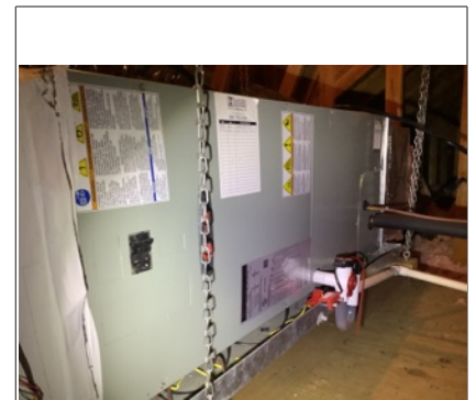
Reference picture of the furnace/blower coil in the attic.
