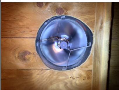
Roof/attic framing, roof sheathing and insulation appeared to be in overall functional condition where accessible.
