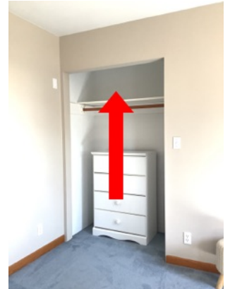
Summary item 1x Missing closet doors were observed in the 2nd floor bedrooms. Recommend installation of replacement closet doors where indicated as deemed necessary.
