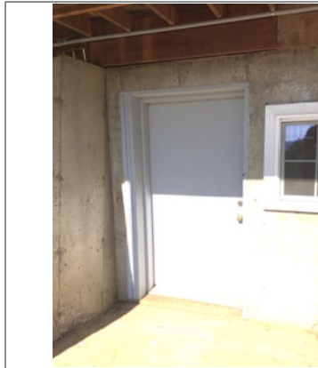
The exterior doors appeared to be in overall functional condition unless noted.
