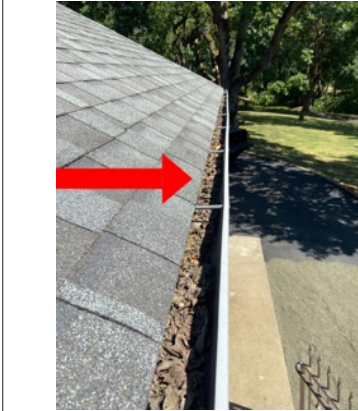
Summary item 1c Debris was observed at the interior of the gutters and downspouts around the perimeter of the home. Plugged gutters/downspouts may lead to moisture intrusion into the crawl space/basement and could potentially impact the foundation. Recommend clearing any/all debris from the gutters and downspouts to promote proper roof drainage. Recommend observing the perimeter drainage for additional signs of blockage and perform cleaning maintenance as needed.
