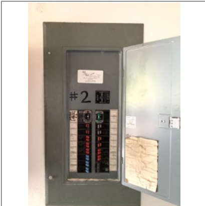
Reference picture of the electrical panel box.
