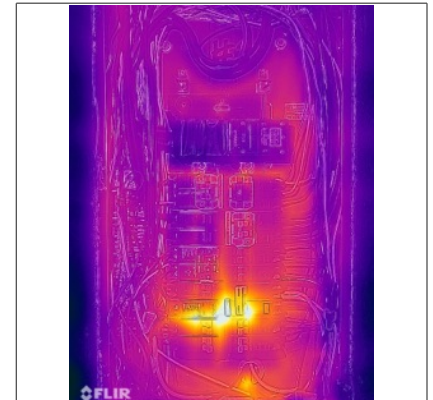
Infrared image of the electrical panel box/wiring. No signs of overheating were evident with an infrared camera, thermal probe and visual inspection.
