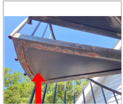
Summary item 1 Rust/corrosion was observed at the steel frames at the exterior spiral staircase. It would be recommended to treat the steel frames at the exterior spiral staircase with a rust inhibitor and perform painting maintenance to prevent further deterioration. Inspections and maintenance should be ongoing.
