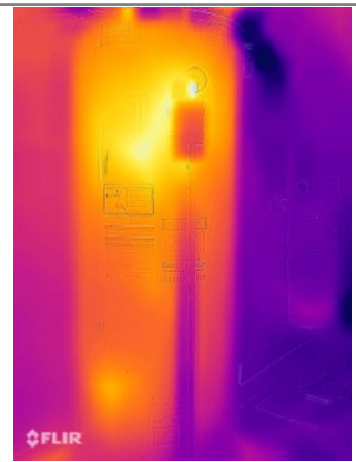
The water heater appeared to be functioning properly at time of inspection. Hot water was effectively delivered to all necessary points throughout the home.
