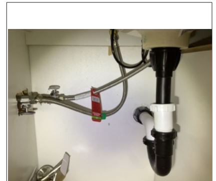
No active water leakage was apparent at time of inspection unless noted.
