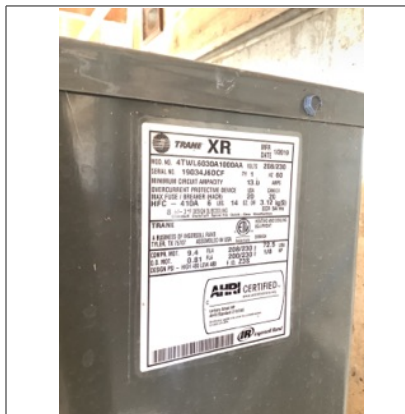
Reference picture of the heat pump rating label.
