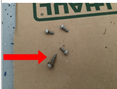
Summary item 7a Two of the screws at the electrical sub-panel box cover have pointed ends which are not rated for electrical panels. Recommend replacing screws with blunt ended screws rated for electrical panel box covers.
