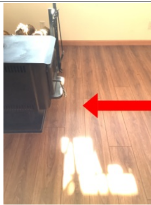
Summary item 1m The wood stove was installed without a hearth pad which could allow for embers to damage the flooring in front of the wood stove.
