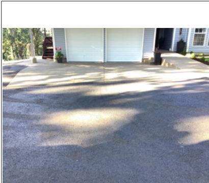
The driveway appeared to be in overall usable condition. Typical cracks were observed at the concrete driveway. Recommend sealing cracks to prevent further deterioration.
