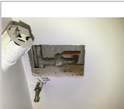
Reference picture of the primary water shut off valve in the basement
