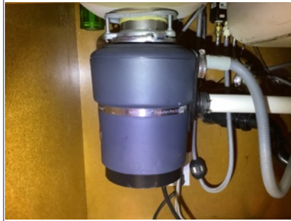
The garbage disposal was tested and appeared to be functional.
