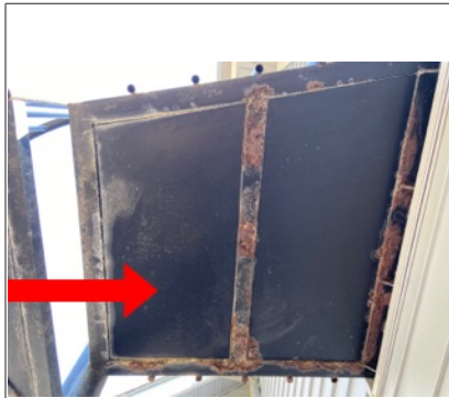
Summary item 1 Rust/corrosion was observed at the steel frames at the exterior spiral staircase. It would be recommended to treat the steel frames at the exterior spiral staircase with a rust inhibitor and perform painting maintenance to prevent further deterioration. Inspections and maintenance should be ongoing.
